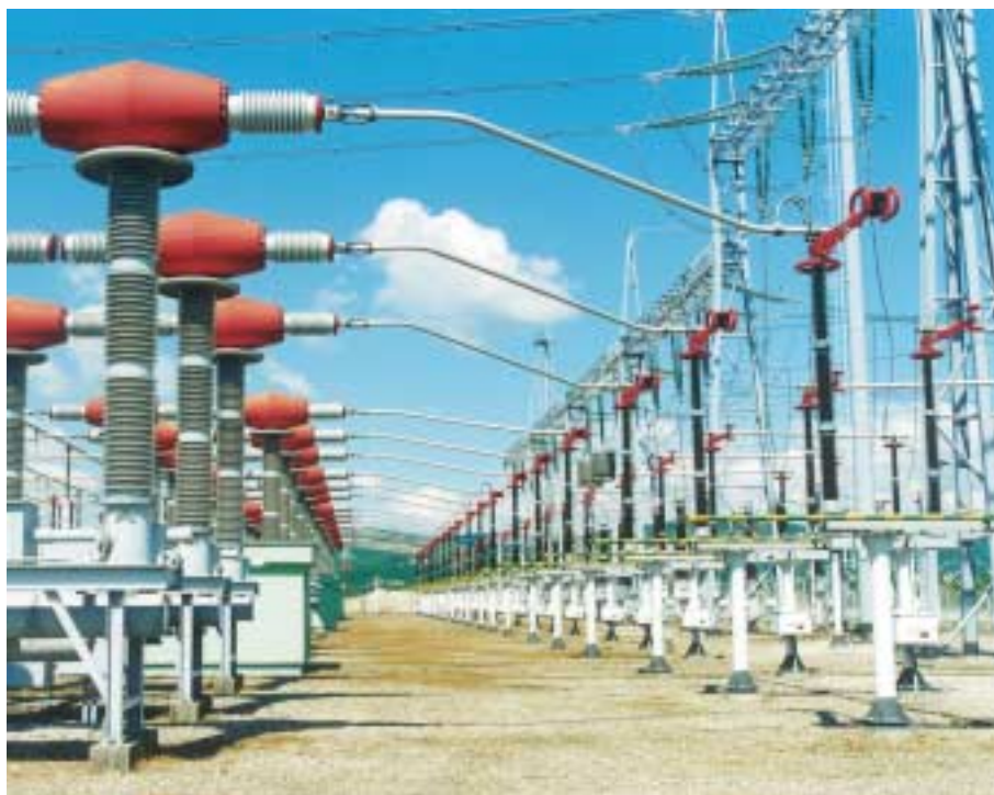
Switchyard of the Krško NPP.
